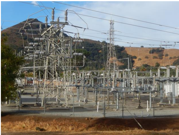
Morgan Hill Substation
